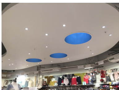
Fig. 7 – Photo of the light tube solution in demonstration area
