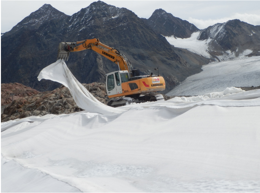
Figure 4 – Workers use a digger for removing geotextile covers in summer 2015. Copyright 2015 by H. Nöbauer.
