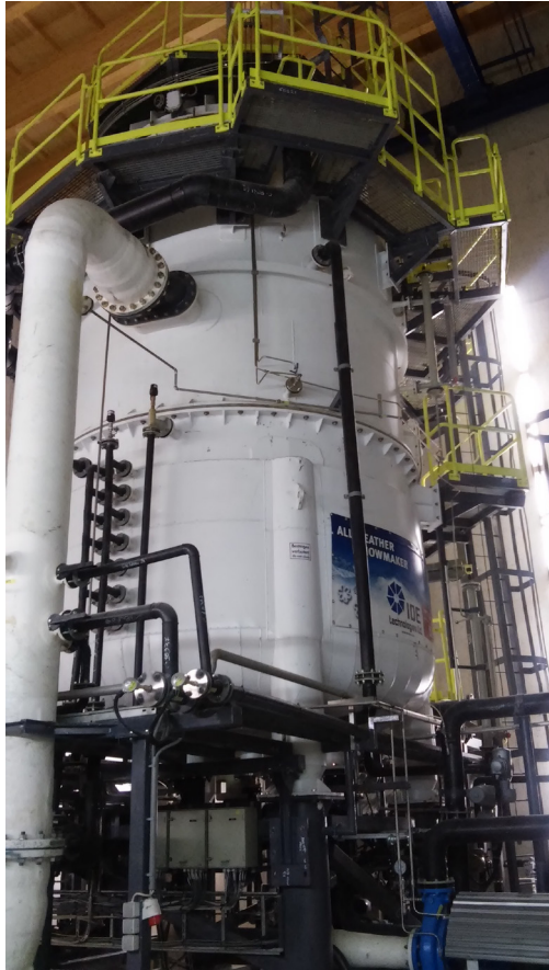
Figure 2 – The All Weather Snowmaker installed inside a special building. Copyright 2016 by H. Nöbauer.
